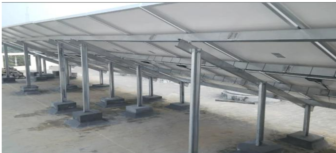
Solar panel mounting structures
